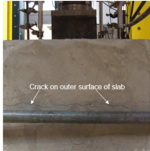
Figure 9. Longitudinal cracks on outer surface of a slab observed from test specimen M6
