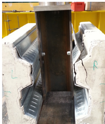
Figure 10. Deck de-bonding in left slab and rib shear failure in right slab of specimen M2
